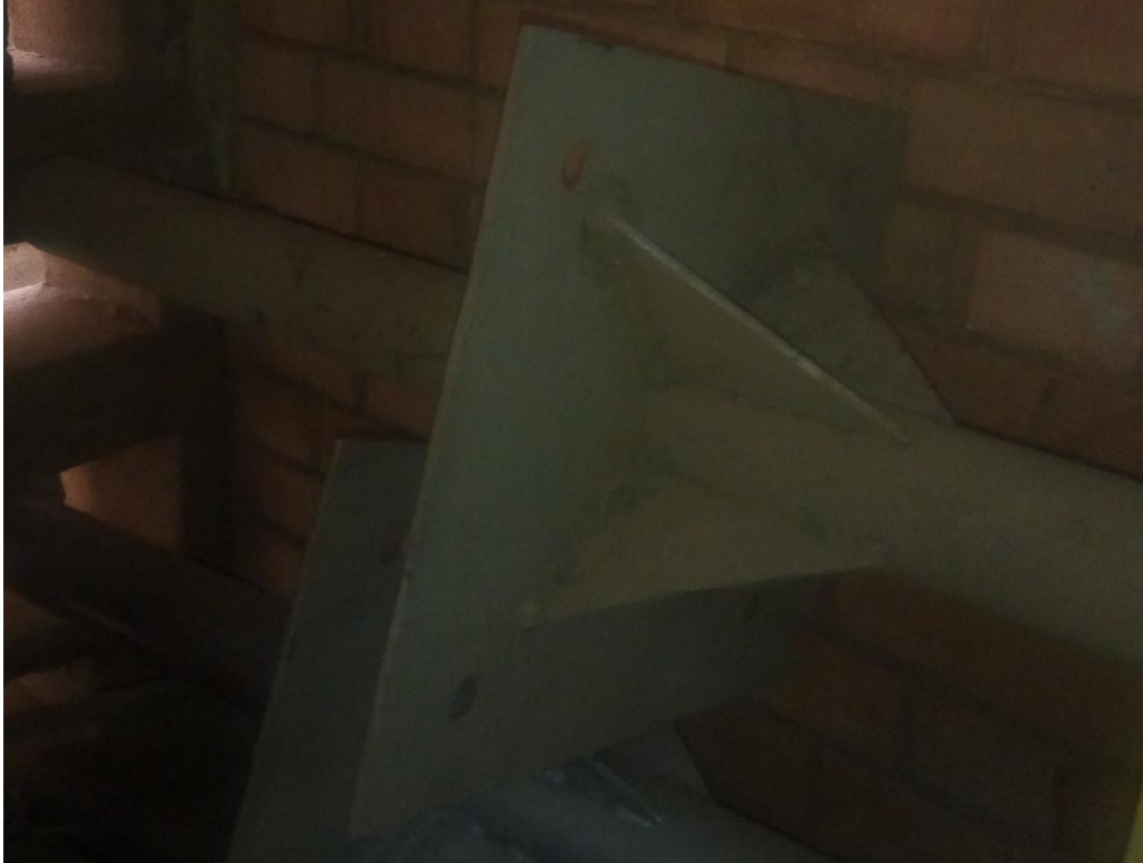
Figure 4. Metal plate that separates the area to go below and above the ground
